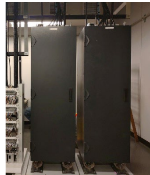
CBTC wayside equipment
